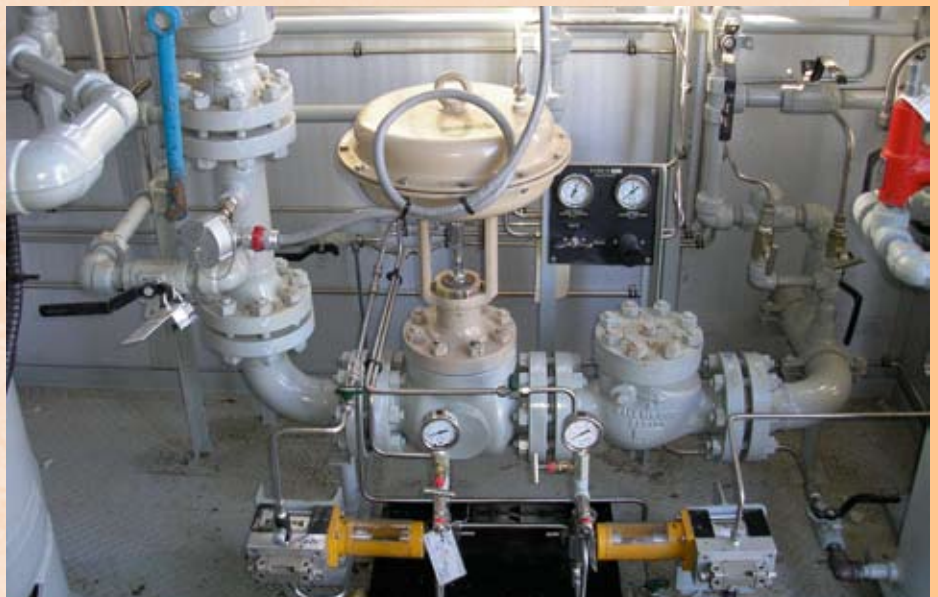
A SAMSON Type 3251 Control Valve provides back pressure control on a natural gas separator.
