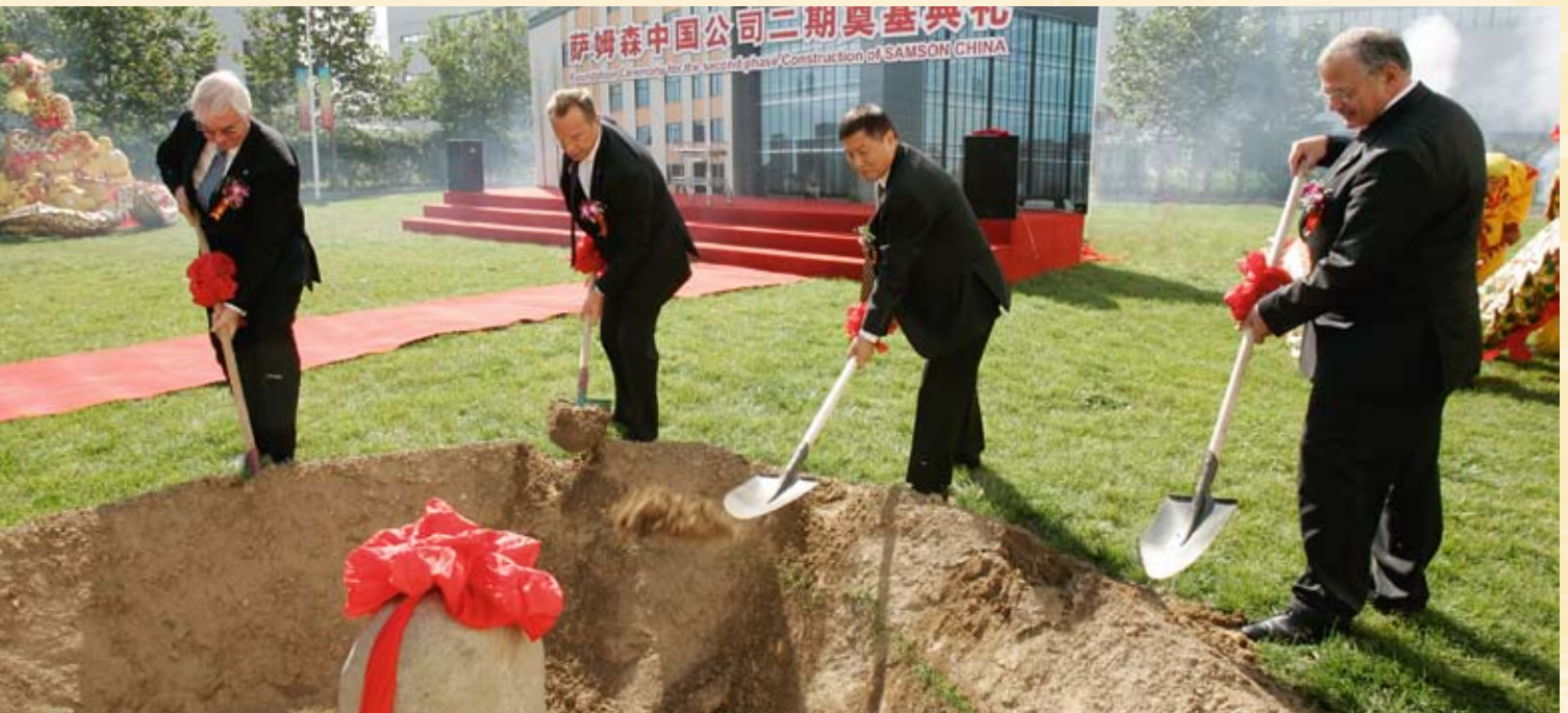
Hans-Erich Grimm (head of the Sales Division), Dr. Nikolaus Hensel (Chairman of the Supervisory Board), Ying Tao Zhang (head of SAMSON China) and Ludwig Wiesner (Chairman of the Executive Board) laid the foundation stone for the new SAMSON building in Beijing.
