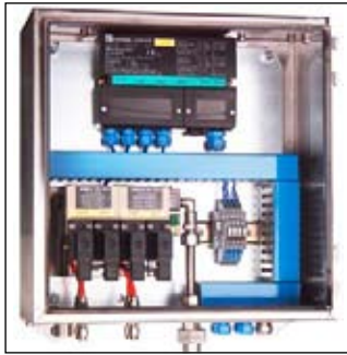
Fig 10: Fieldbus control unit including four on/off valves
