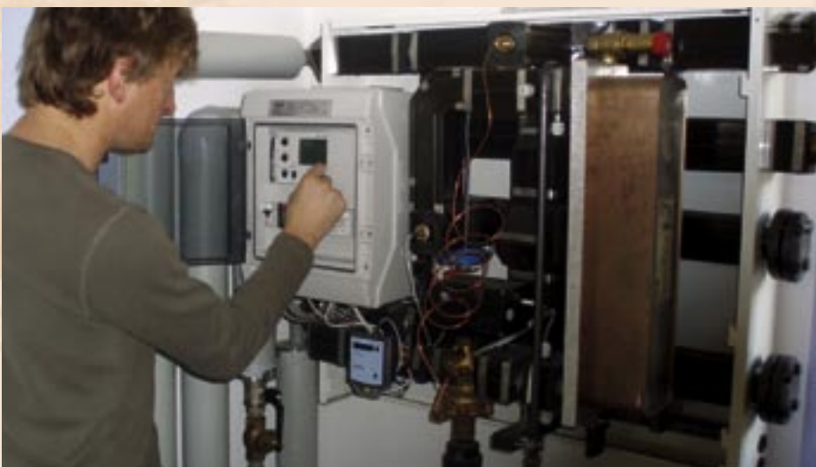
Instead of boilers, homes and hotels have their own transfer stations.
