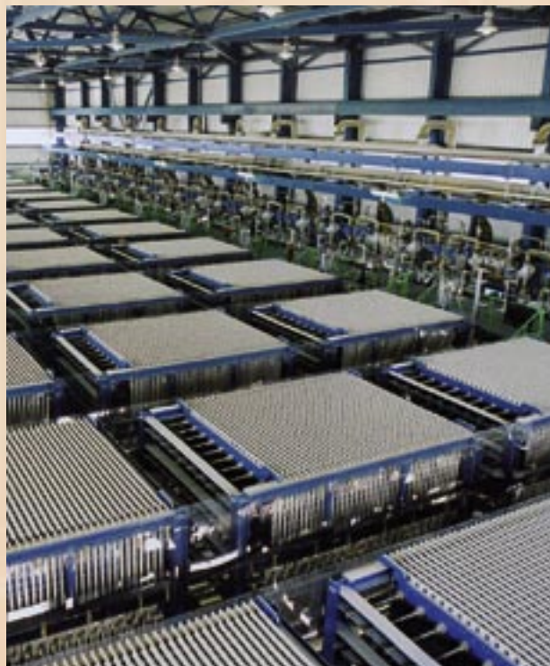
Large amounts of hydrogen are released in the cell hall of a chlorate factory during chloro-alkali electrolysis.
