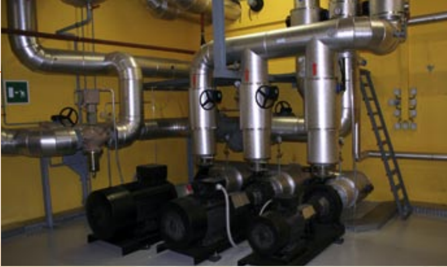
Pumps transport hot water to the individual transfer stations.
