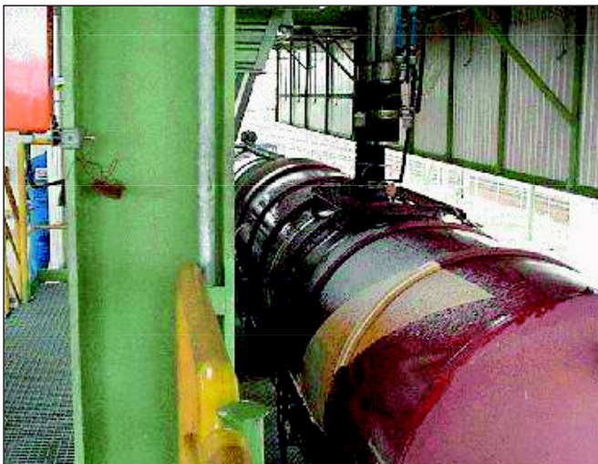
Fig. 25: Petrol loading station: Too small sizes of rotary valves on first floor cause noise and severe dangerous pipe vibration
