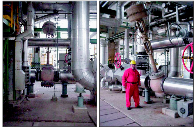
Fig. 18: Installation problems solved
